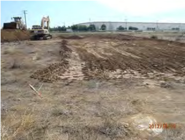
Looking South along East side of excavation with OU1MW21 in the foreground
