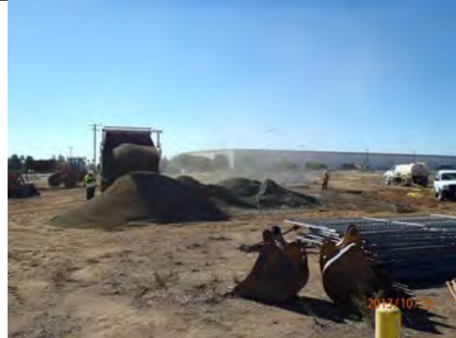
Importing soil from West Coast Sand and Gravel for backfilling the excavations.
