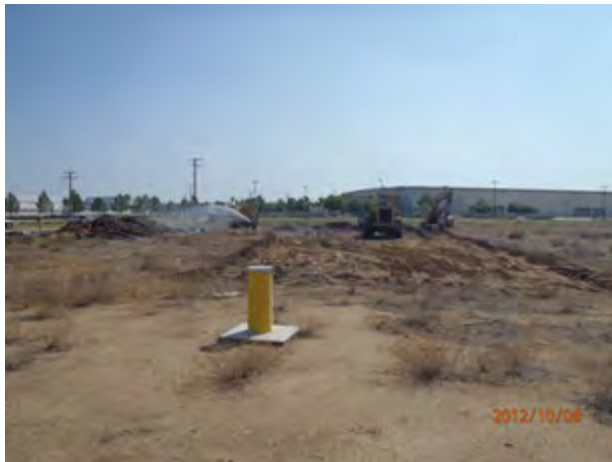
Excavating Site FT-007, looking South with 7MP03 and OU1MW-21 in the for ground
