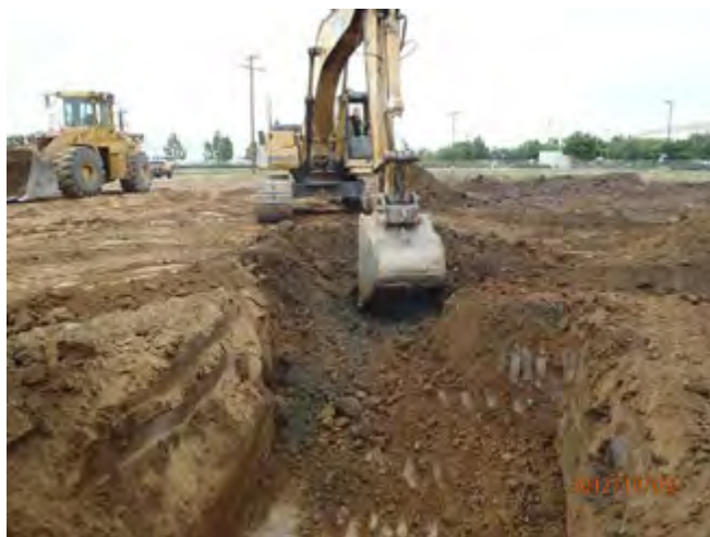
Excavating and removing gray soils down to brown soil with very low odor levels.
