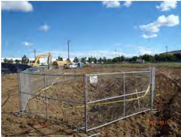
Looking South at the deeper excavation area secured using the chain linked fence
