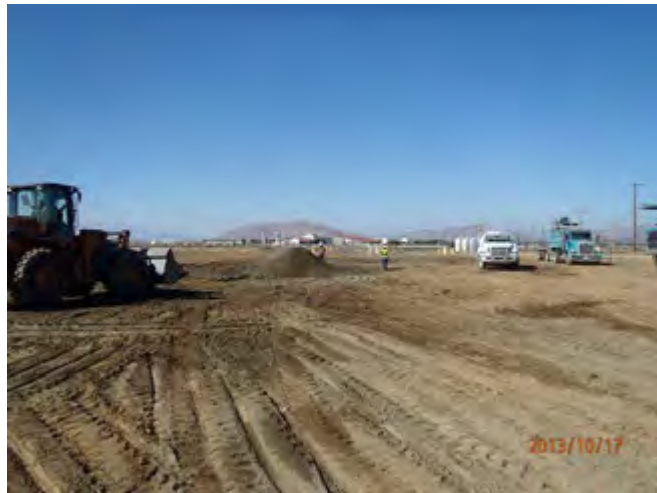
Soil conditioning and compacting excavation with Norcal performing soil compaction testing, Looking North
