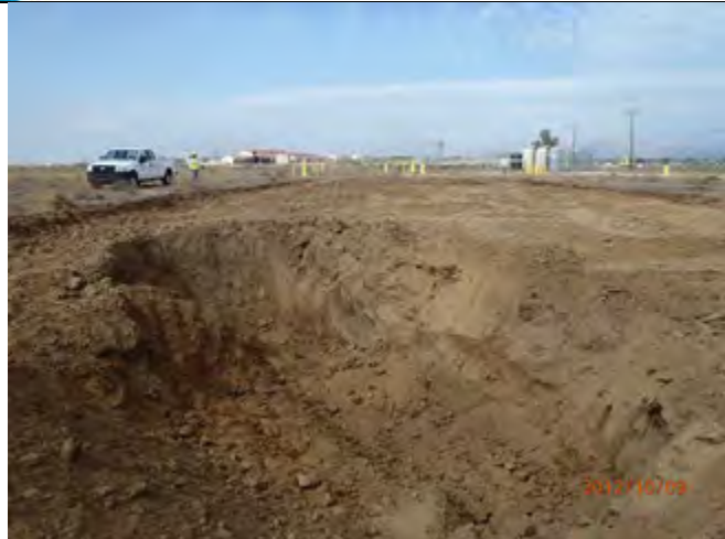
Hot spot area excavated out to brown soil, gray soil max depth observed was 6 feet
