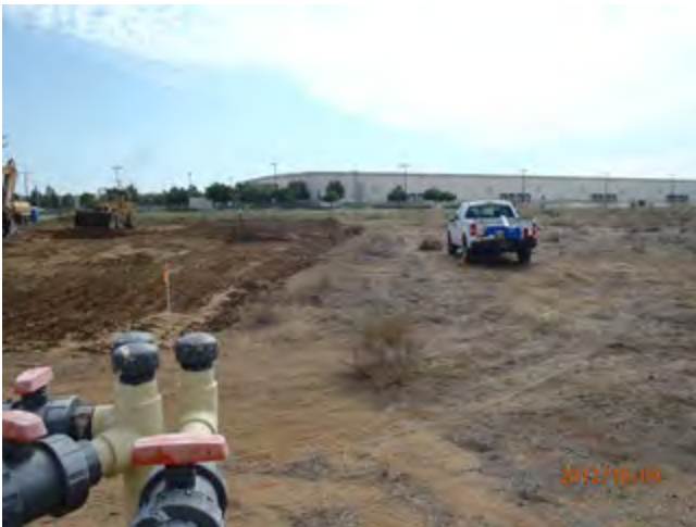
Looking South along West side of excavation with 7SVE02 in the foreground
