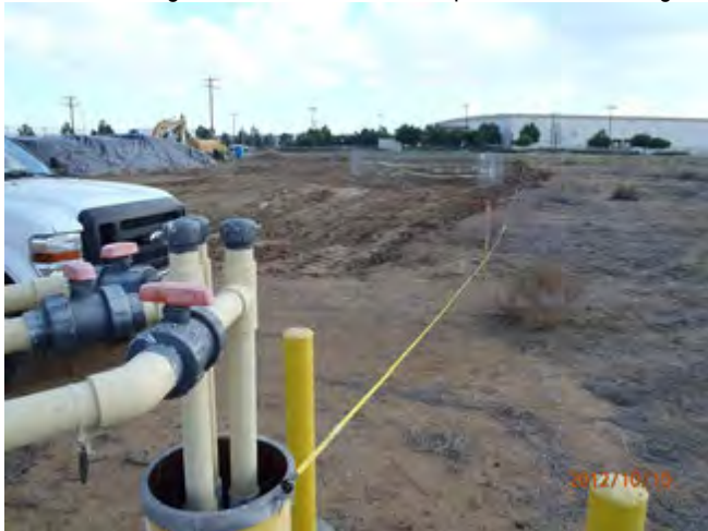
Looking South from 7SVE02 with measuring tape used to grid out site for confirmation sampling
