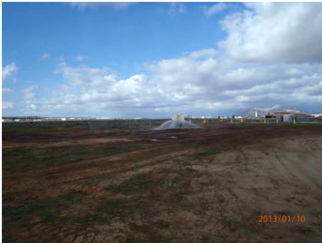
Wet site down to create a dirt crust to help prevent dust and to enhance grass growth
