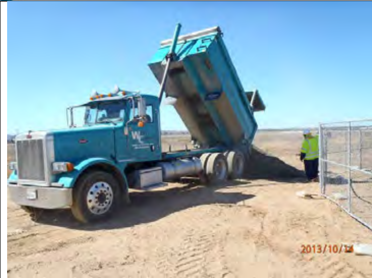
Importing soil from West Coast Sand and Gravel for backfilling the excavations.
