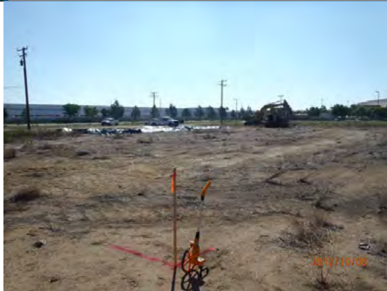
Site FT007 grubbed, looking south from the NW corner of the excavation area
