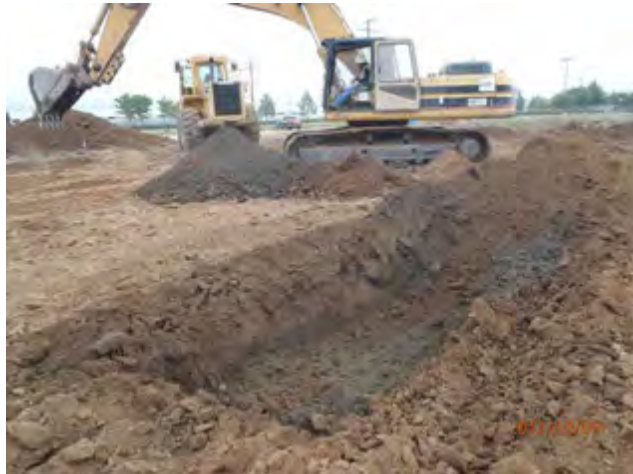
Located hot spot of grayish soil with low PID reading average around 15 to 20 ppm
