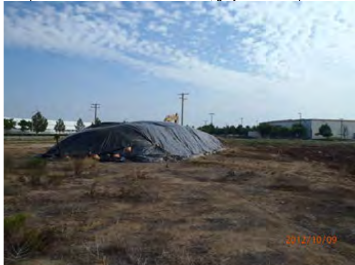
Stock pile approx. 8x25x70 feet = 518 cu yards, covered and secured awaiting analytical results
