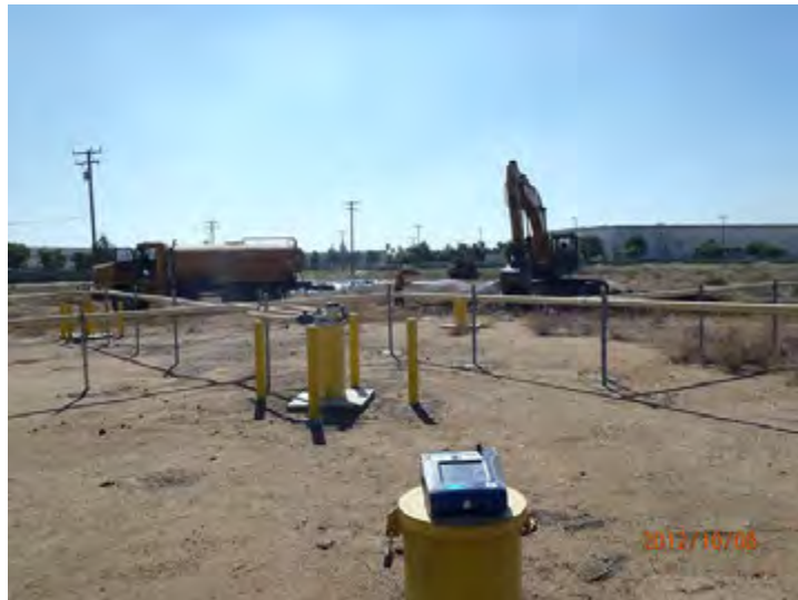
Dust Trak II dust monitor located down wind, looking south from 7MP02
