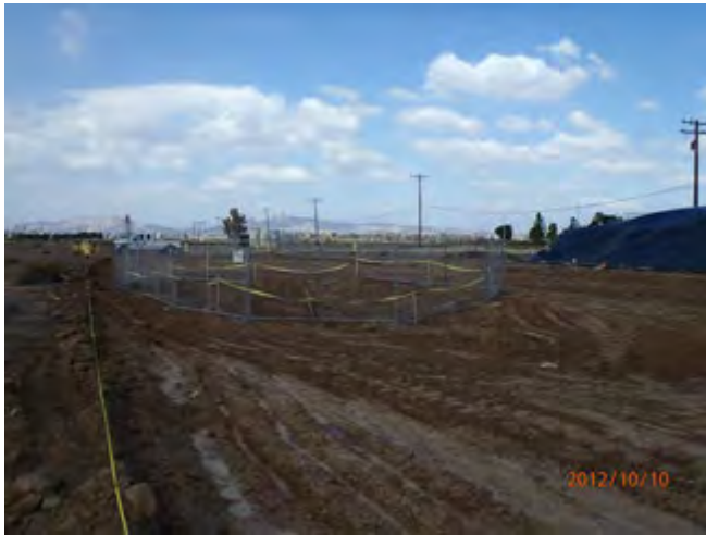
SW area looking North at the secured deeper excavation using the chain linked fence
