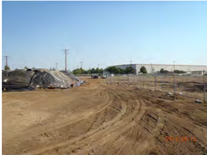
From NE corner of site looking South over secured excavation areas and secured Stockpile.
