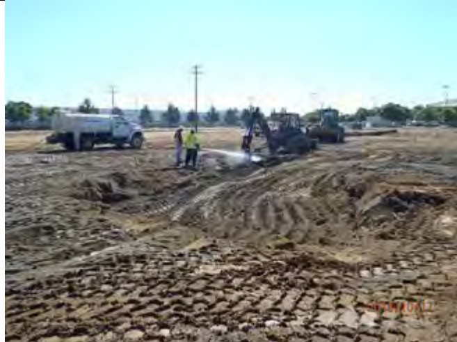
Soil conditioning and compacting excavation with Norcal performing soil compaction testing, Looking South
