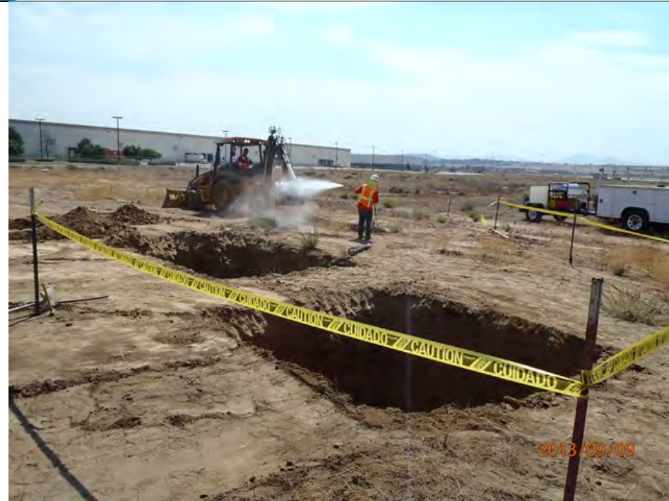
From NE corner of site looking South West at excavation and dust control work
