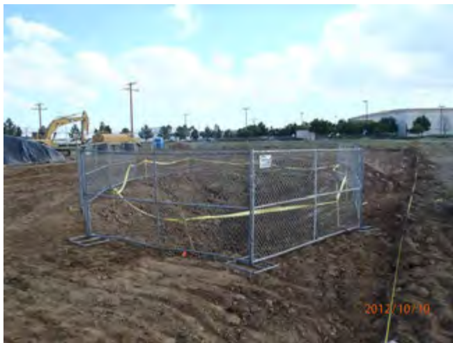
NW area looking South at the secured deeper excavation using the chain linked fence
