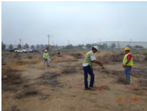
Crew marking out FT007 excavation area, looking south from the NW corner of the excavation area
