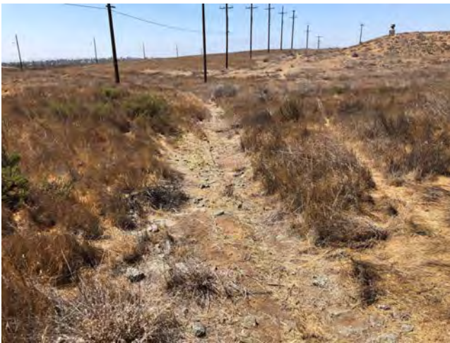
Photo 15. Downstream view of Abandoned Drainage (AD-1), where flows historically commenced at the culvert (Photo 15) (33.906067, -117.311156). August 6, 2021.
