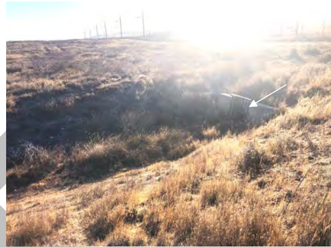
Photo 6. Culvert (white arrow) through which flows enter the more defined and wider portion of NWW-3, facing east. Based on field observations and a review of aerials, flows likely originated from within the bunker area via a storm drain inlet (similar to Photo 5) (33.908661, -117.312008). August 6, 2021.
