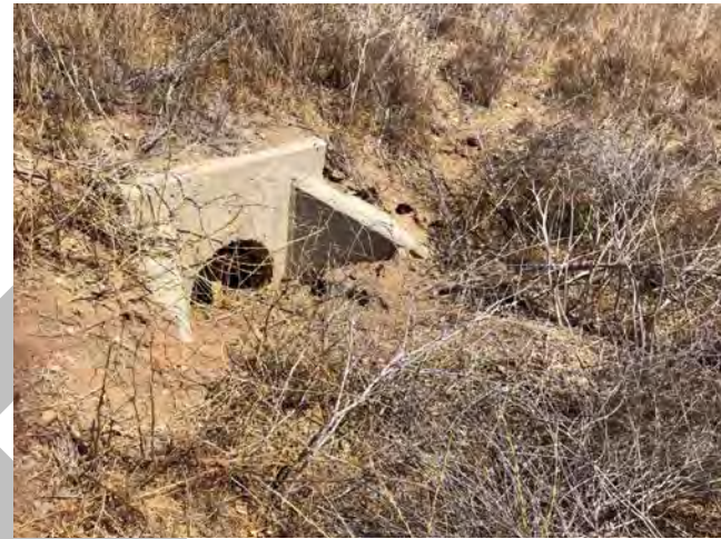
Photo 10. View of culvert, facing southeast, that historically provided flows to NWW-3 through a storm drain inlet. This culvert was representative of the other culverts within the bunker area that historically provided flows to the storm drain inlets (33.904439, -117.311138). August 6, 2021
