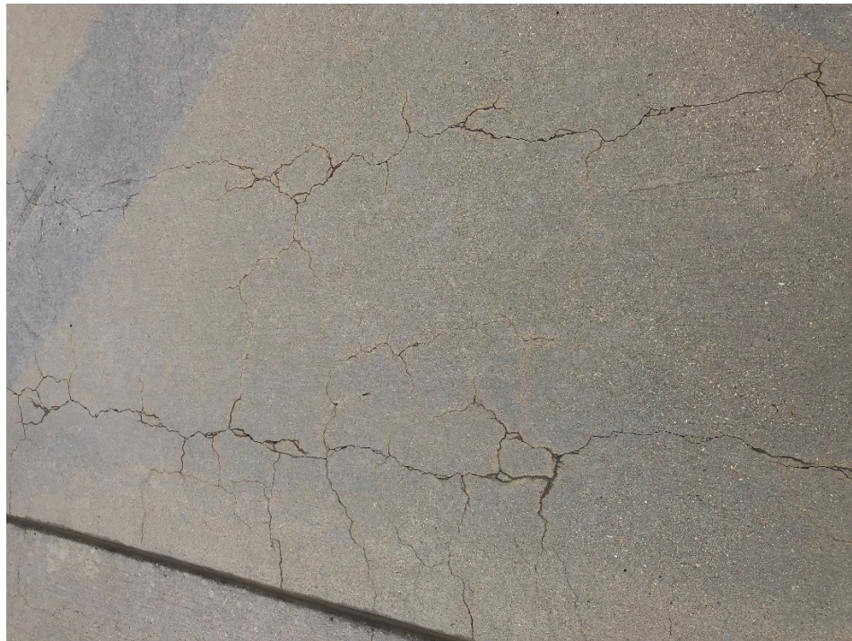
Photo 11: Alkali Silica Reactivity, ASR (medium severity)
