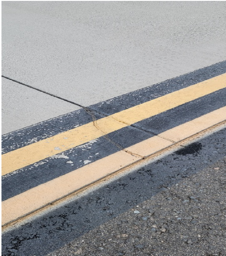
Photo 13: Corner Spall (low severity)
