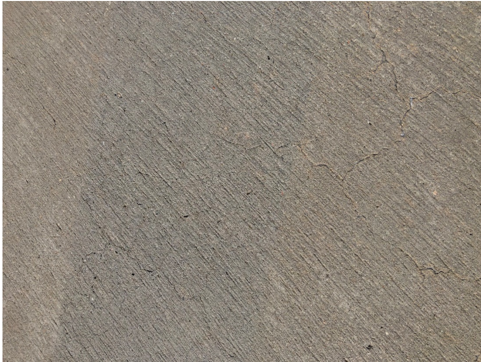
Photo 10: Alkali Silica Reactivity, ASR (low severity)
