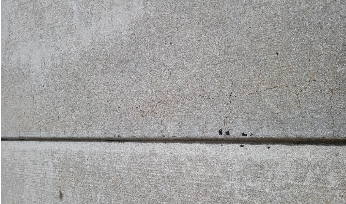
Photo 9: Durability Cracking (low severity)
