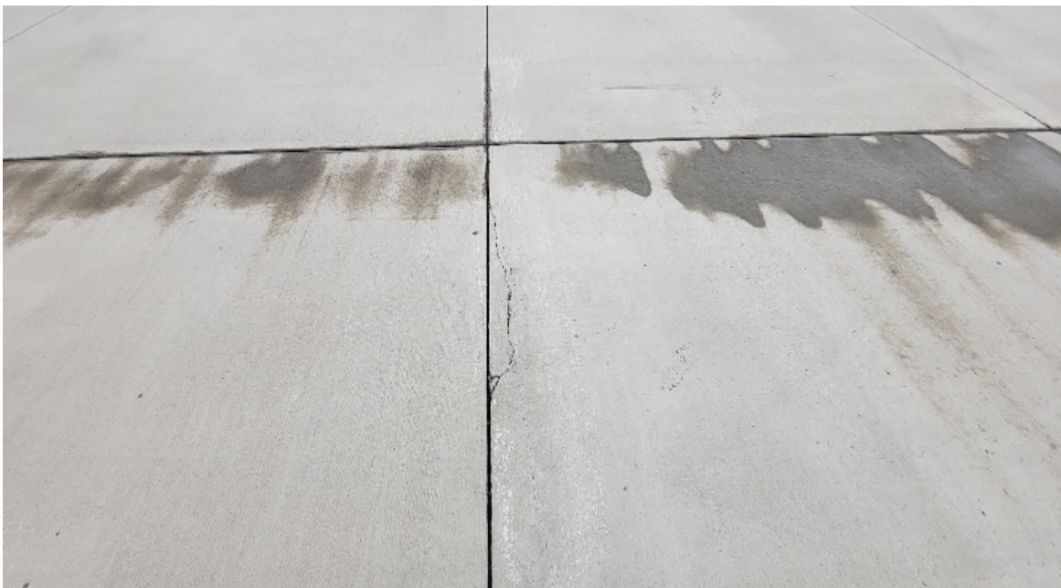
Photo 15: Joint Spall (medium severity)
