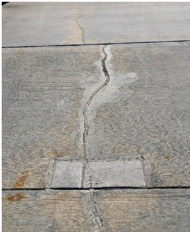
Photo 2: Longitudinal/ Transverse Cracking (Medium)
