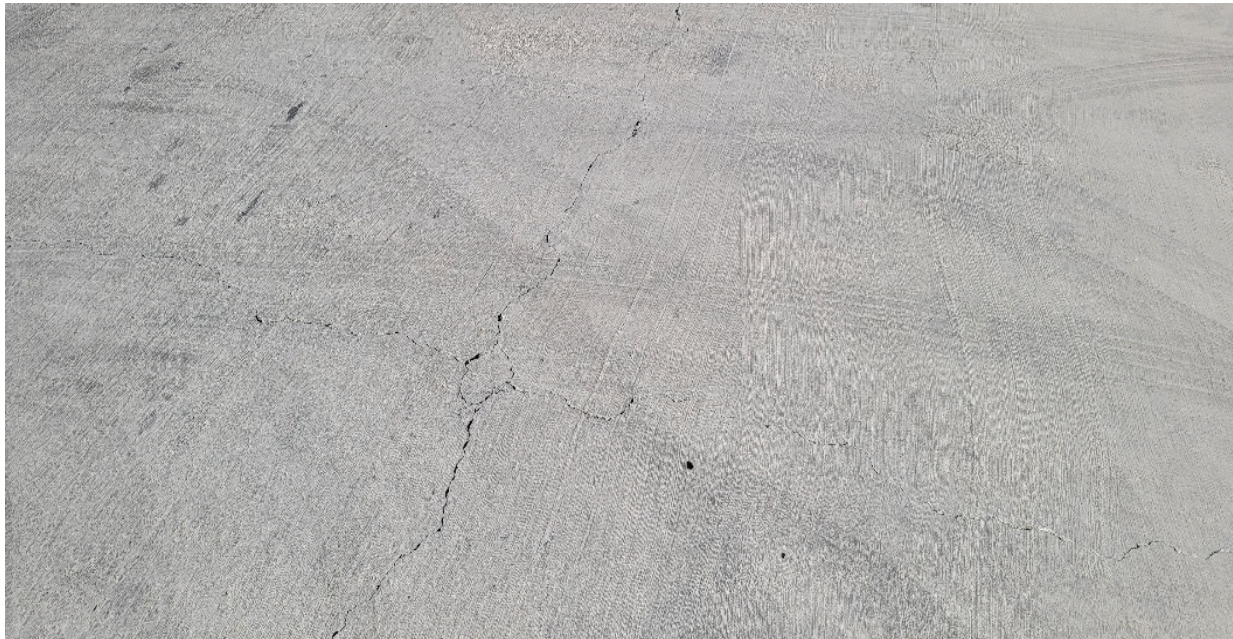
Photo 6: Shattered Slab (medium severity)
