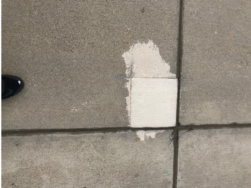
Photo 3: Small Patch (low severity)
