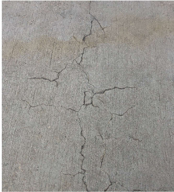
Photo 1: Longitudinal/ Transverse Cracking (low severity)
