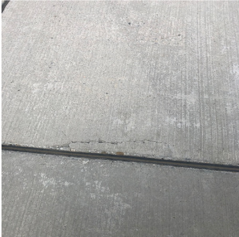
Photo14: Joint Spall (low severity)
