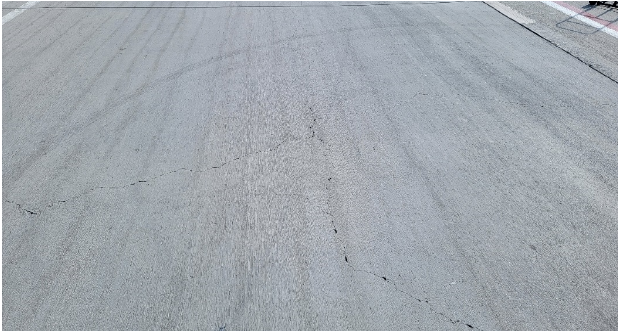
Photo 5: Shattered Slab (low severity)
