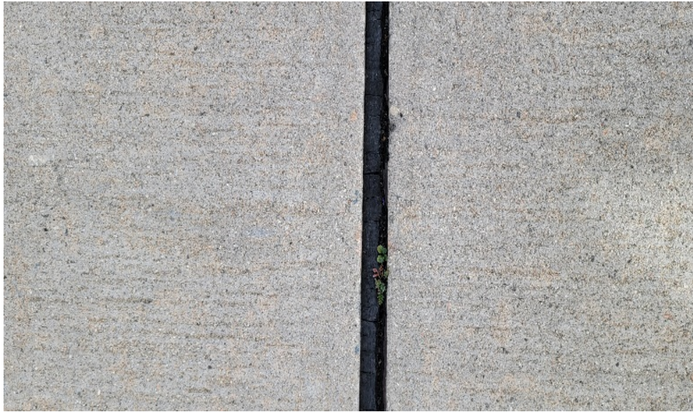
Photo 7: Joint Seal Damage (medium severity)
