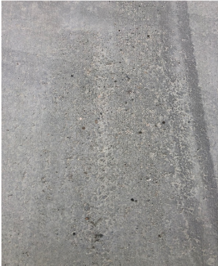
Photo 12: Scaling (low severity)
