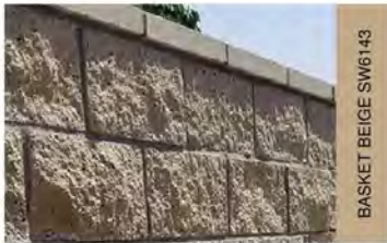
6' HIGH MASONRY WALL WITH WALL CAP- TO BE PAINTED BASKET BEIGE ON SIDE TO BE MAINTAINED BY LLMD
